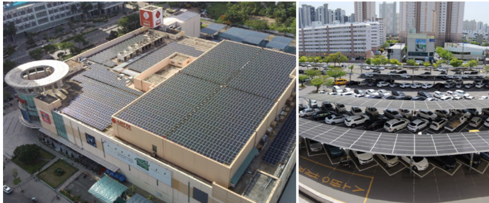
Solar power facilities at LOTTE Mart
