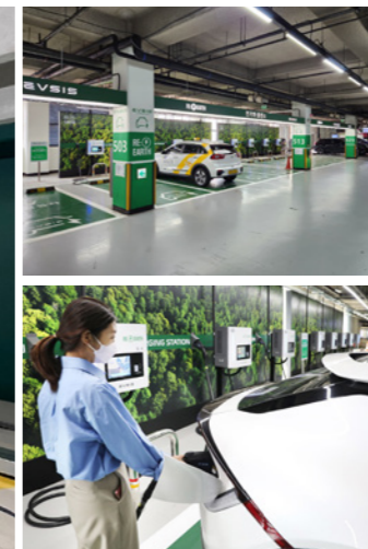
EV Charging Station at LOTTE Mart Gyeongang
