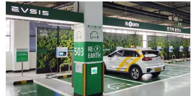
EV Charging Station at LOTTE Mart Gyeongang
