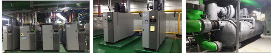
<Installed boilers at the Daegu Store>
