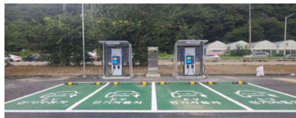
Charging Station for Electric Vehicles
