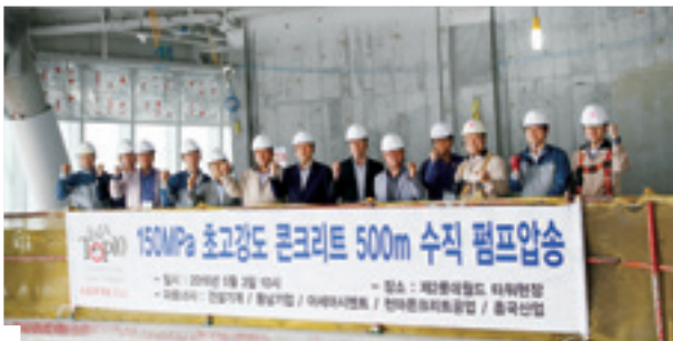
The site where the UHSC vertical pumping was successful for the first time in world at 150MPa*
