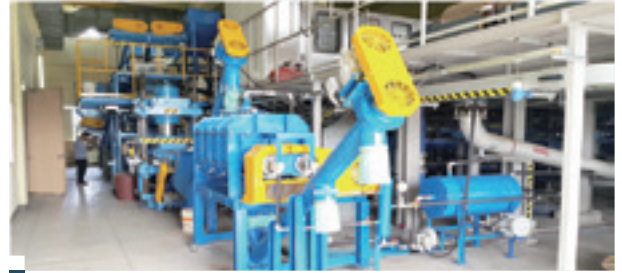
An organic waste drying and fueling plant being researched for commercialization
