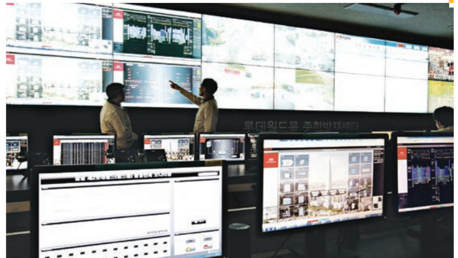
24-hour integrated control center
