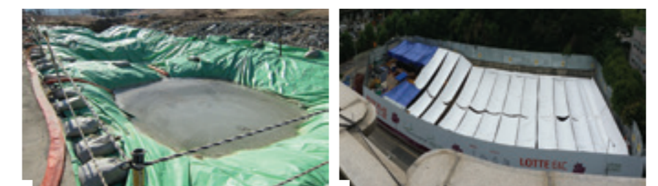
Water management by installing multi-stack sedimentation facilities
