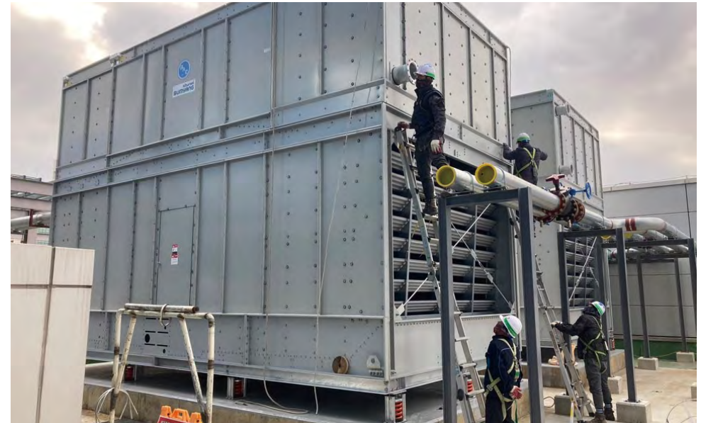
Cooling tower for free cooling
