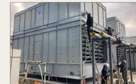
Free cooling system
