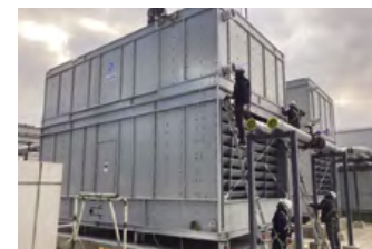
Cooling tower for free cooling
