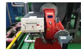
Low NOx burner in the 1st data center
