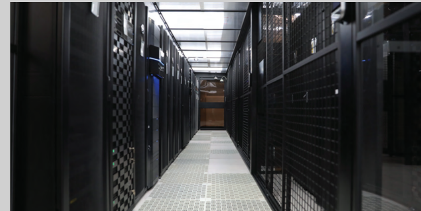
Cold Aisle Containment System
