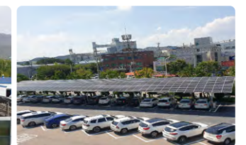
Solar panels at parking lots
