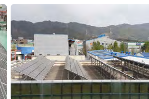
Solar panels in the packaging section
