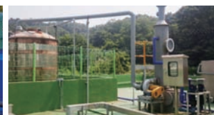
Washing-type Dust Collector System
