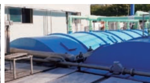
Waste Water Treatment Equipment
