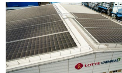
LOTTE Chemical Vietnam Corporation solar power plant
