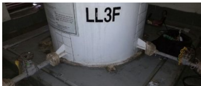
Sulfuric Acid Tank's Leak Detector in the Daesan Facility
