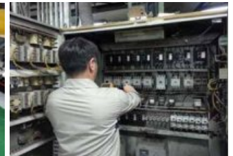
Support for Partner Companies CASE 2 (KWANG JU FISHING NET): Safety Inspection and Repair of Electrical and Instrumental Equipment
