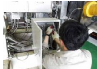
Support for Partner Companies CASE 1 (EALTECH): Replacement/Repair of Aged Equipment
