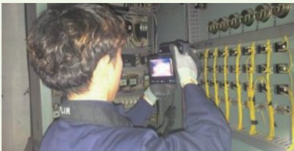
Inspection of KOMAX Industrial
