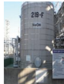
Daesan Plant: Flow prevention bump for storage tank
