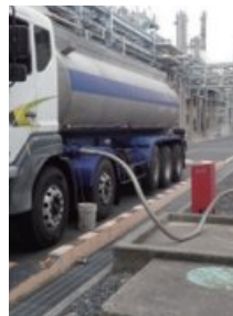
Yeosu Plant: Flow prevention bump for tank lorry
