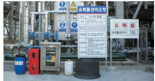
Hazardous Chemical Substance Leak Prevention Equipment
