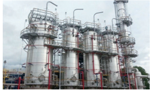
Lotte Chemical's Titan TBA Plant in Malaysia
