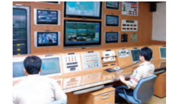
Emergency Protection System
